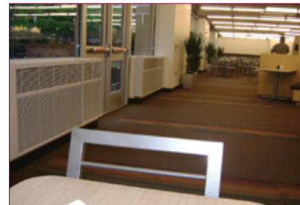
Figure 14: DV diffuser with integrated heat installed along the perimeter
