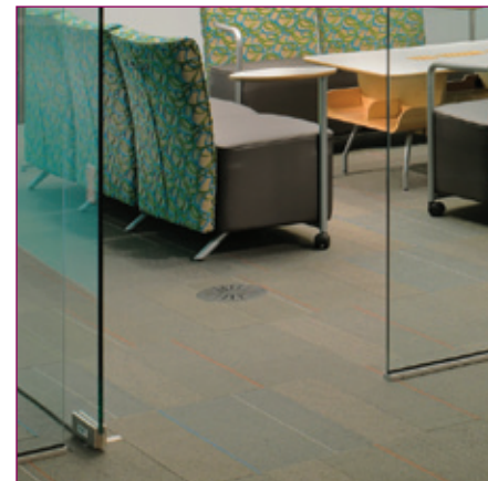
Figure 30: RFDD installed in floor
