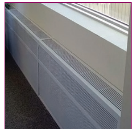
Figure 28: DLE-H installed against wall
