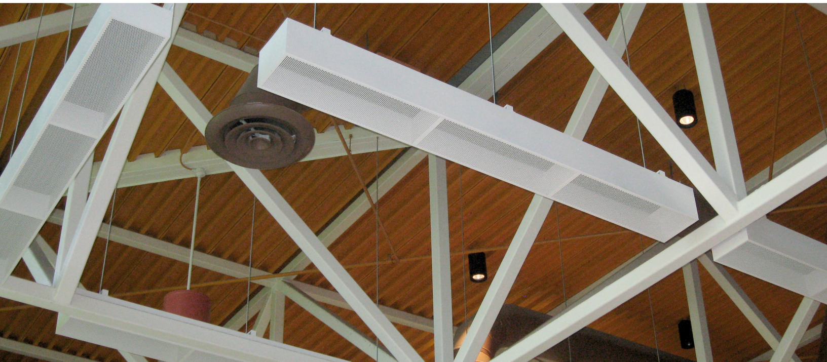
Open ceiling application
